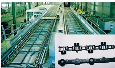
"MEP Chain" Conveyor Adoption of operator-centric free flow system where products stop in front of operators
